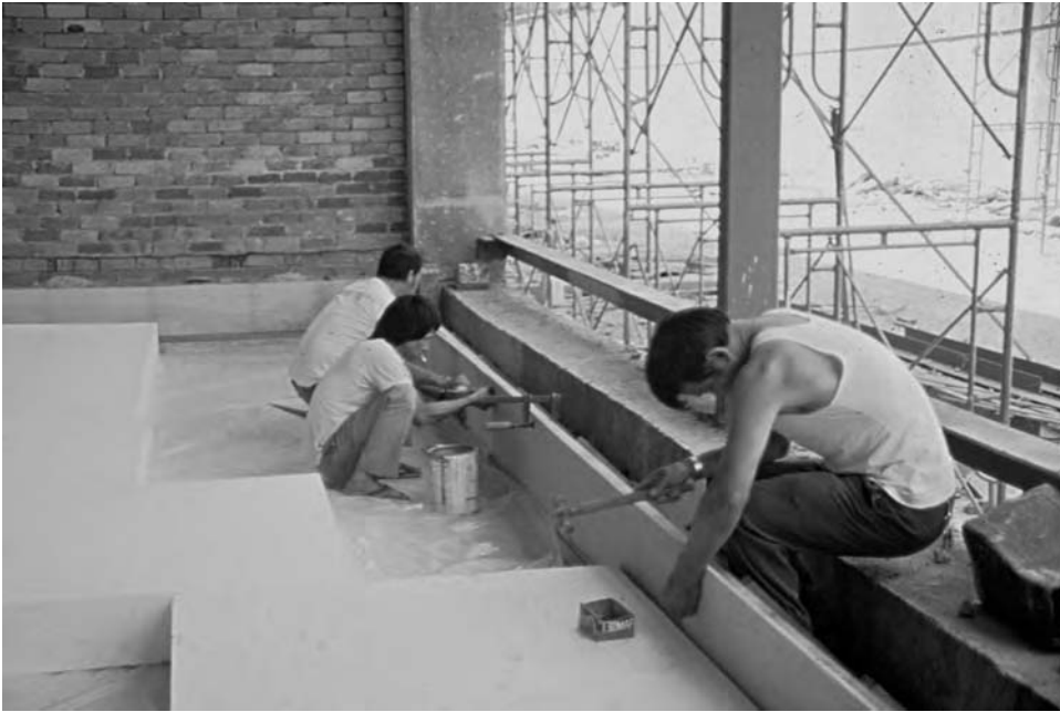
Figure 4.1 Freezer floors usually include a thick course of insulation under the slab
