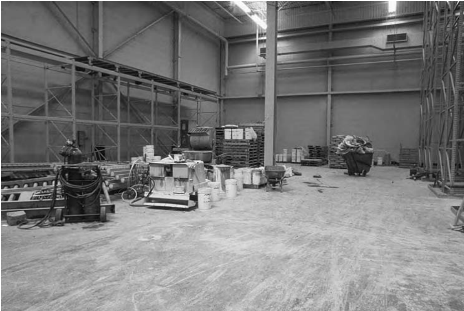
Figure 20.1 Premature wear on an industrial floor
