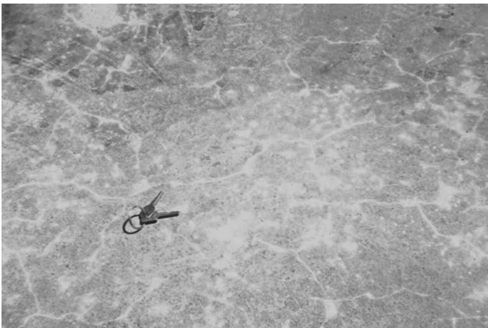
Figure 13.2 Craze cracks don't look pretty, but rarely cause real harm
