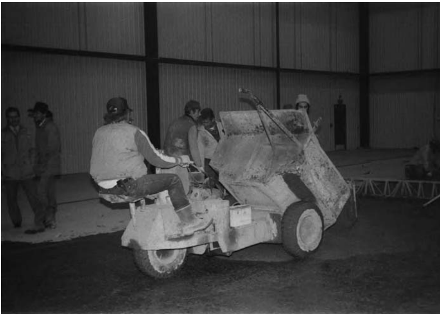
Figure 11.2 Using a power dumper (buggy) to place concrete for a thin, bonded topping
