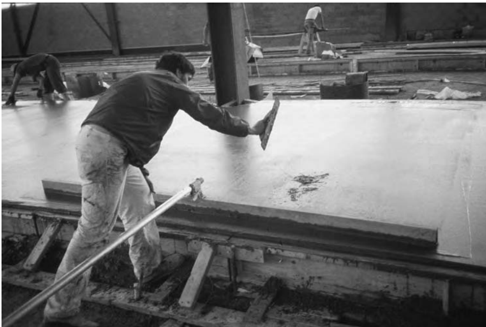
Figure 19.8 Superflat construction – filling a low spot that the highway straightedge has revealed
